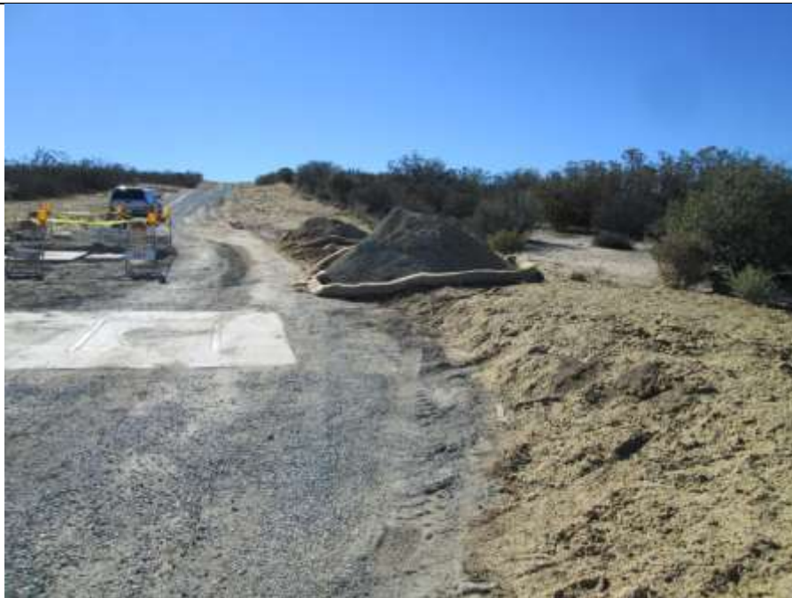
Photo 2: Erosion and sediment control devices (straw wattles) were observed implemented around stockpiles (MM-HYD-1) during construction along the 138 kV underground line.
