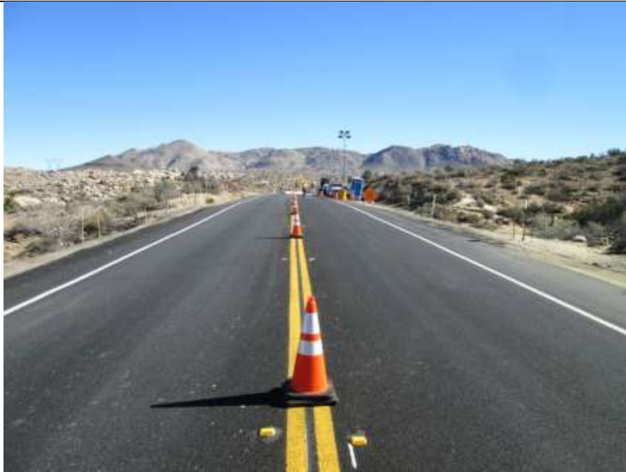
Photo 1: Traffic control measures consisting of traffic cones, signs, and flaggers were observed being utilized to direct motorists along Carrizo Gorge Road during work activities in accordance with MM-TRA-1.
