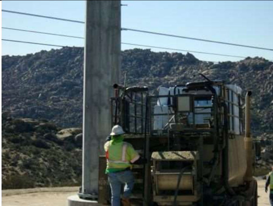
Photo 3: During hydroseeding along the pad slopes of temporary work areas along the 138kV overhead line, crews were observed carrying required fire equipment in work vehicles in accordance with MM FF-1.
