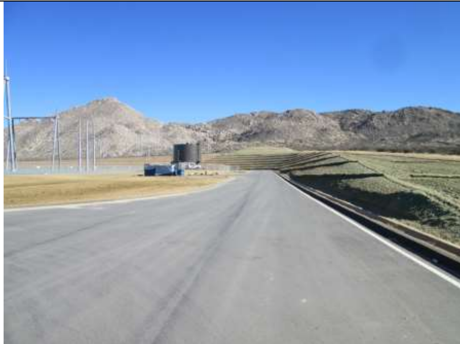
Photo 4: Restoration activities at the ECO substation this reporting period consisting of applying approved hydroseed mixtures on slopes adjacent to the substation. Slope stabilization BMPs, including straw wattles, were observed to be installed and in working condition(MM-HYD-1).
